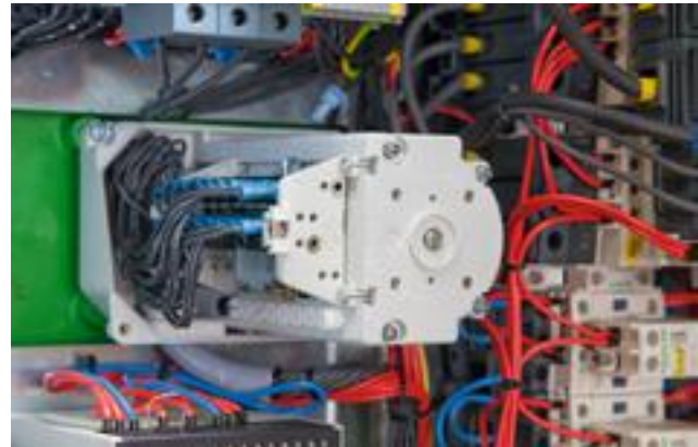
Emergency hoist limit switch (gear limit switch)
